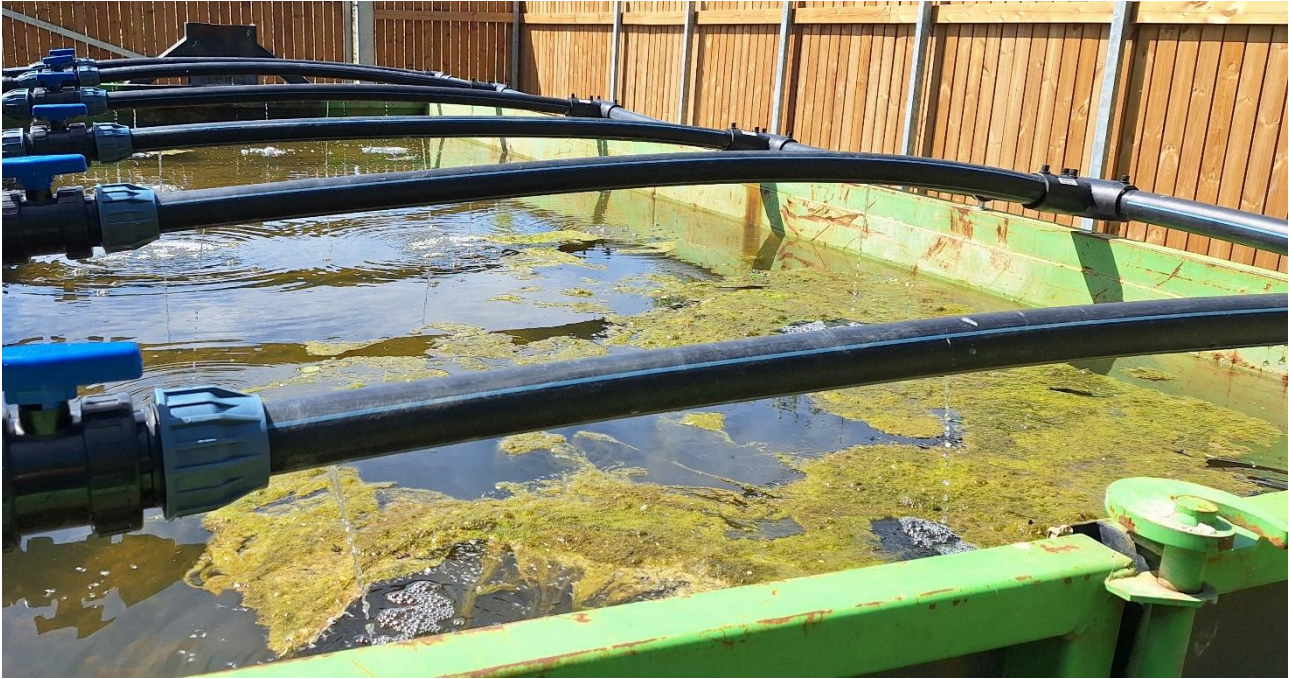
Figure 6. Extensive biomass growth observed in the crushed limestone filter at the end of the sampling campaign.
