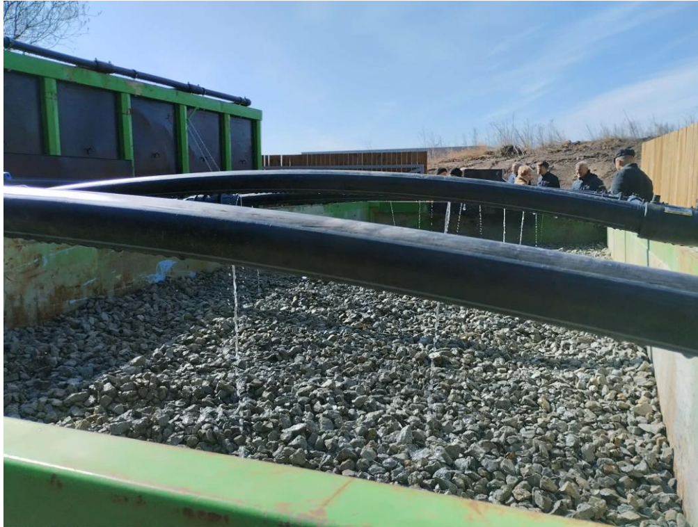
Figure 4. The filtration system during operation.
