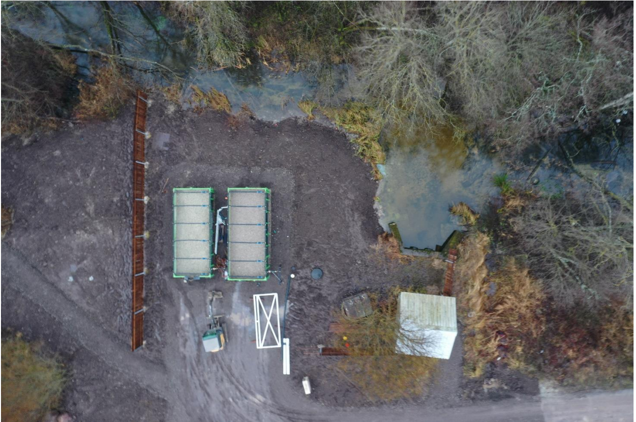
Figure 2. Aerial view of the Estonian pilot site and the filtration system.
